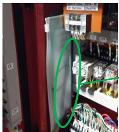
The Pump Starter Panel
